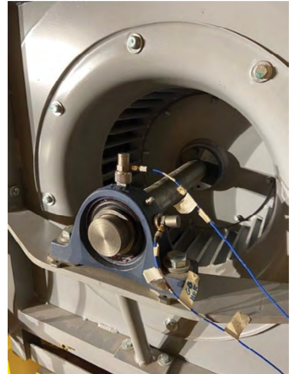
Figure 2: Temporary Accelerometers Mounted on the Fan Outboard Bearing Casing
